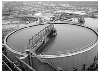
Sludge wastewater treatment plant (WWTP).
